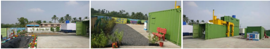
Fig. 2 Plant photographs of thermal FSTP
