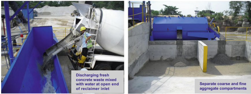
Fig. 5 Typical view of recycling of fresh concrete waste (reclaimer)
