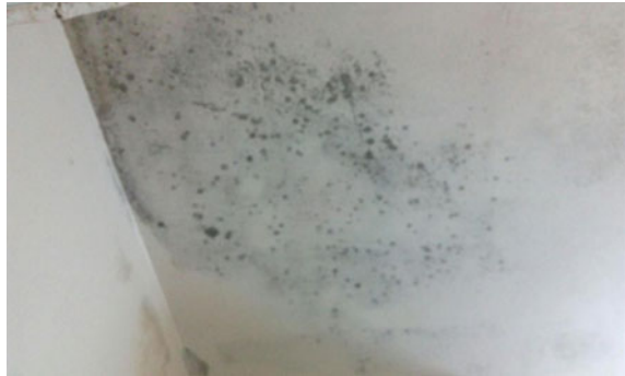
Fig. 30.2 Wall of an air-conditioned room showing microbial growth due to dew formation due to the direct impact of primary air from adjacent room unit
