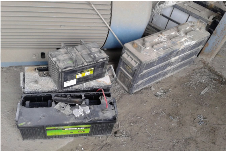
Fig. 4 Unsafe storage of scrap batteries
