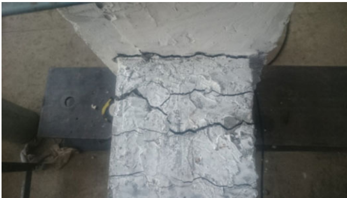
Fig. 10 Specimen failure before retrofit
