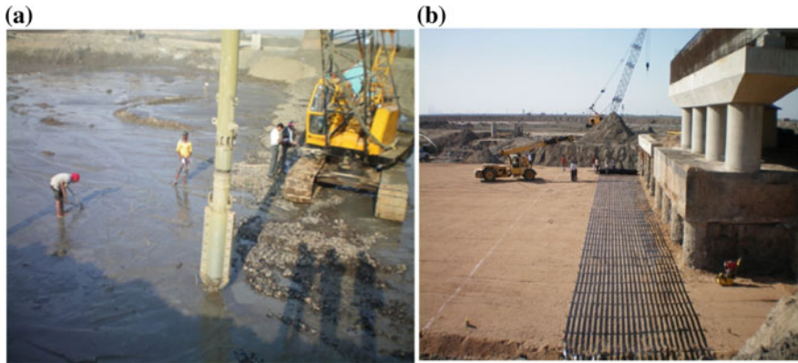
Fig. 7 During construction a installation of stone column, b laying of high strength geogrid
