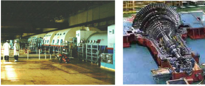
Fig. 5.18 Steam turbine generator unit
