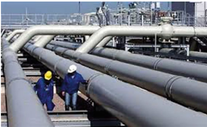
Fig. 1 Visual inspection of damage water pipeline
