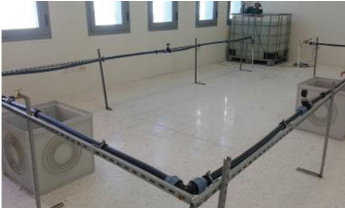
Fig. 4 Testbed water pipeline demonstrator
