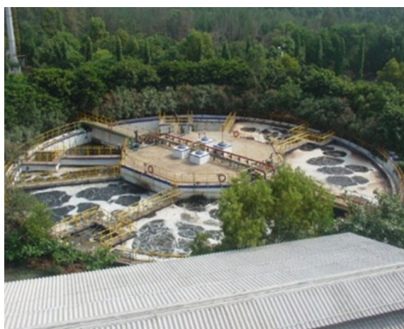
Fig. 21 Effluent treatment plant
