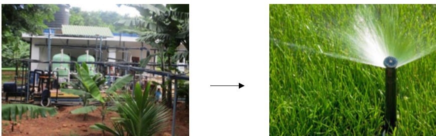
Fig. 10 Sewage treatment plant, treated sewage water used for plantation
