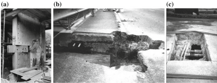
Fig. 8 Damage scenarios carried out in the Z-24 Bridge: pier settlement (a), failure of anchor heads (b), and tendon rupture (c)
