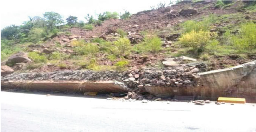
Fig. 8 Landslide due to erosion and reactivates after every rainy season in Murree, Pakistan
