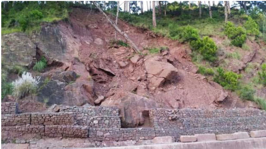
Fig. 7 View of landslide along the road in Murree, Pakistan
