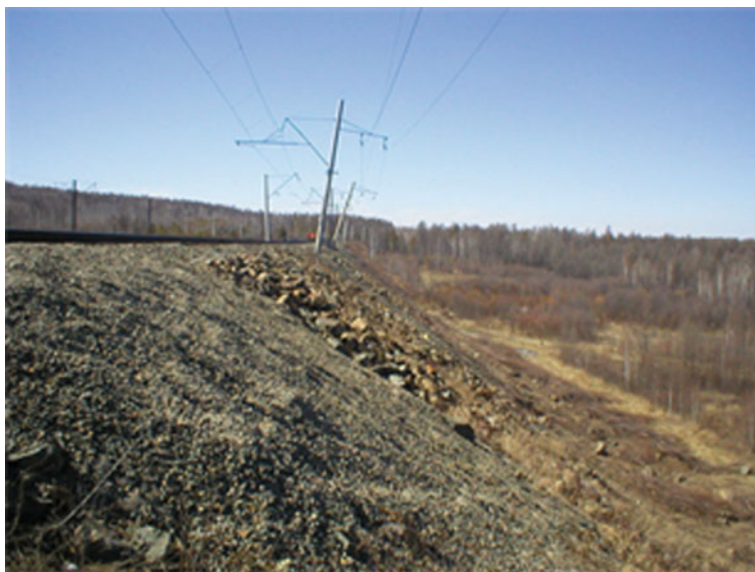
Fig. 1 Deformations of the railway embankment on thawing permafrost soil
