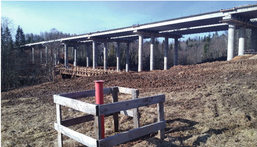
Fig. 1 Point RM47512 geodesic center network for the construction of a bridge across the river Verebushka on PK4751 + 14 highway Moscow—St. Petersburg
