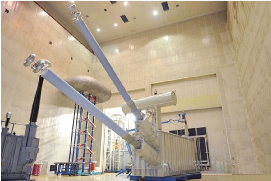
(b) \pm 800 kV UHVDC Converter Transformer (2009)
