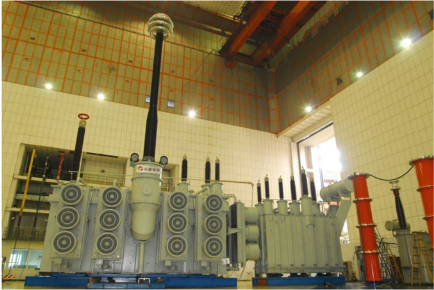
(a) 1000 MVA/1000 kV UHVAC transformer (2008)
