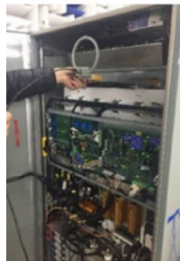
(c) top position of the cabinet
