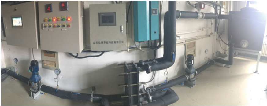
Fig. 5 Indoor equipments of the NRC test rig
