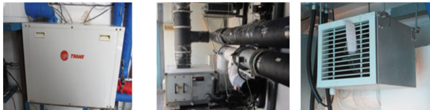
(a) Air-cooled heat pump units (b) Air handling unit (c) VAV terminal unit
