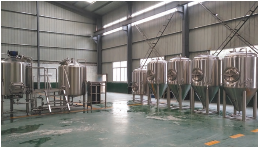
Fig. 6.5 Photo of production workshop
