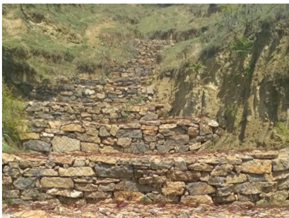
Fig. 3.18 Check dams near Hatiwara, Awantipora J&K
