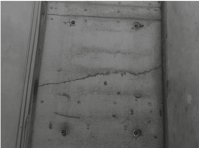
Fig. 2 Restraint cracking on fresh concrete cast in-between two precast members
