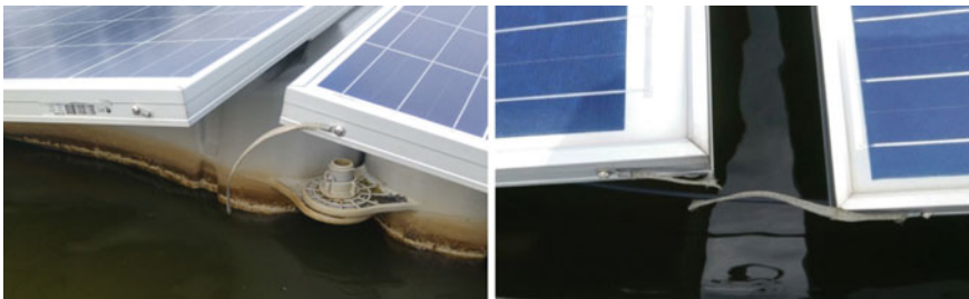
Fig. 9 Examples of breaking and snapping of equipotential bonding tapes (Source SERIS and [14])
