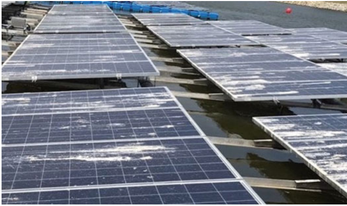
Fig. 8 Severe soiling due to bird droppings in one floating PV system (Figure adopted from [14])
