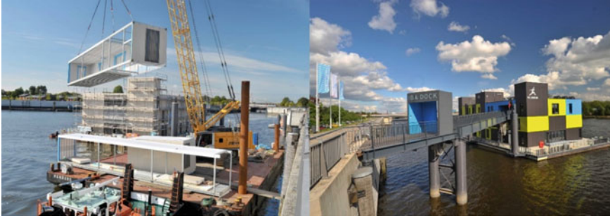
Fig. 6 Constructing modules (left photo); IBA dock (right photo) (photos: Rudiger Mosler) (available at: https://www.archdaily.com/288198/iba-dock-architech , accessed 4 Jan 2019)
