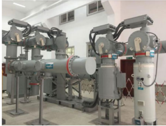
Fig. 9 High-voltage switching device for experiments
