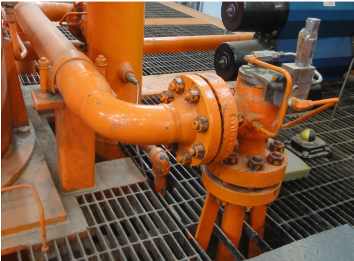
Fig. 1. The first-level outlet safety valve pipe.
