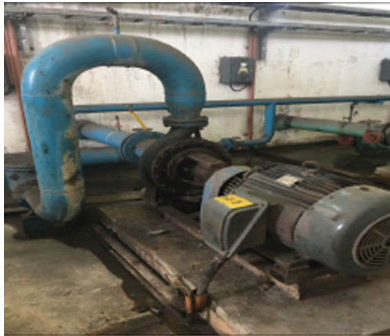
Fig. 8 Targeted pump in Plant B
