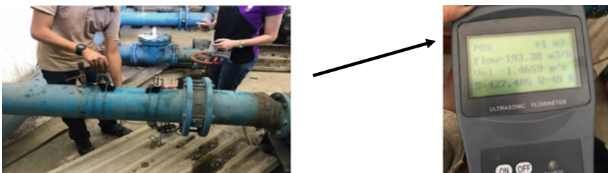
Fig. 13 Installation of flow meter to calculate the flow rate of the pump
