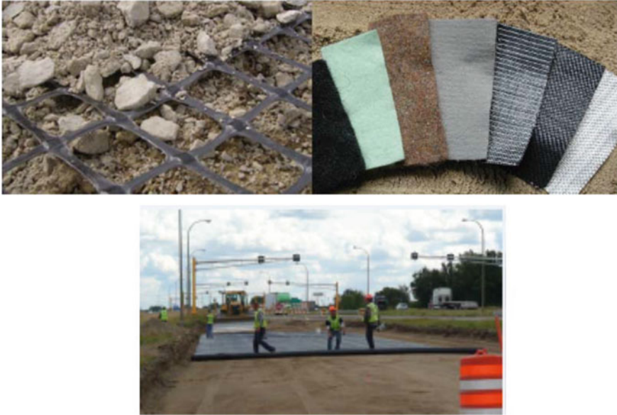
Fig. 6 Top left image shows geogrid reinforcement of a pavement layer, top right image shows woven geotextiles, and the bottom image shows the installation of geosynthetic materials for subgrade layer protection. Source Minnesota Department of Transportation [111]
