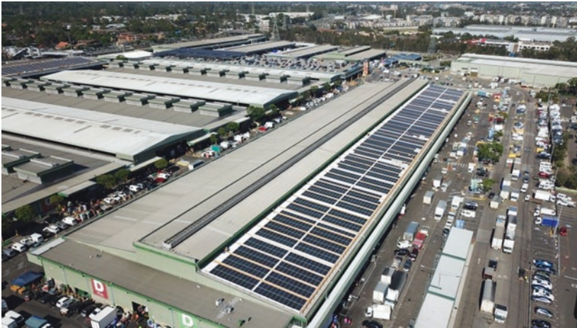
Fig. 3.6 View of part of the 2.2 MW PV rooftop system on Sydney Markets (Source Autonomous Energy (used with permission of Matthew Linney))
