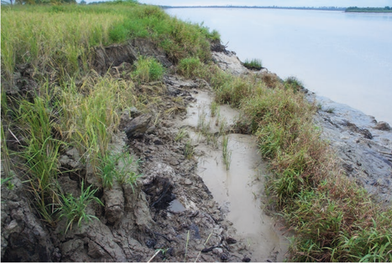
Fig. 2.9 Absence of gravel bars or sand bars along the river channels. (Photograph: Kuniyasu Mokudai 2013)
