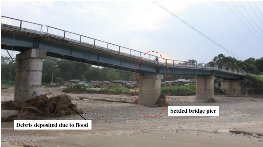
Fig. 4 Dudhaura bridge damaged due to settlement and scouring in Bara district, central Nepal
