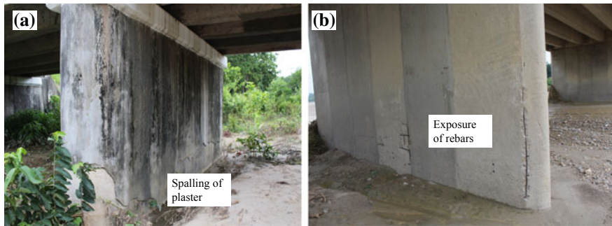
Fig. 3 a Spalling of plaster due to 2017 flood, b exposed re-bar due to flooding
