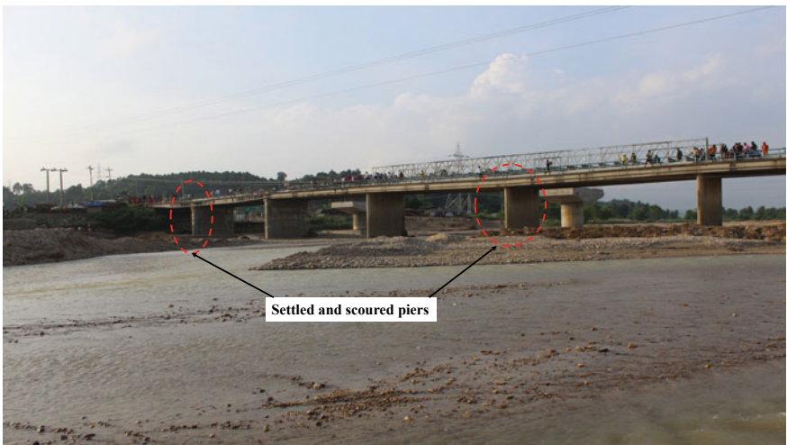
Fig. 5 Ratu bridge damaged due to settlement and scouring in Mahottari district, central Nepal
