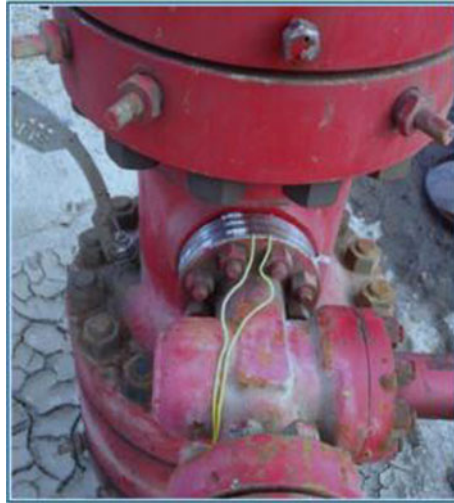
Fig. 5. Photograph of a TCS connection to a wellhead for a pilot survey
