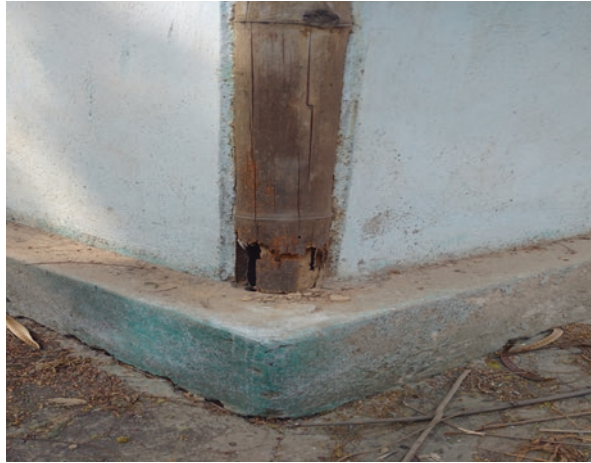
Fig. 6 Decay of untreated bamboo (IIT Delhi, India) in about 5 years of installation
