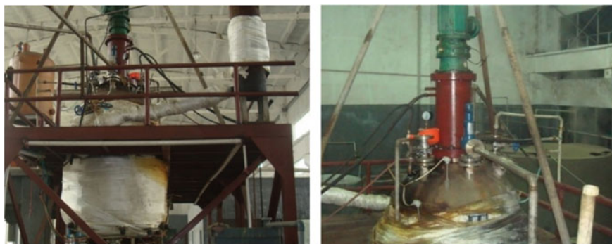
Fig. 5.5 Oxygen pressure alkaline leaching dearsenification pilot-test workshop and autoclave
