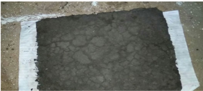
Fig. 4 Dried wall which is almost cracked and no longer in use after a period of 3 months and no watering
