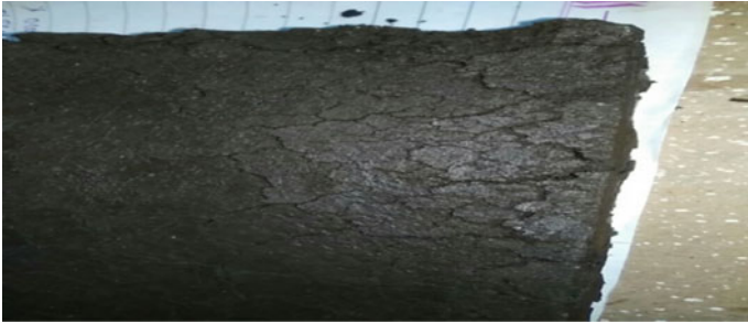
Fig. 3 Initial development of cracks in wall after an interval of 4 months without maintenance but periodic watering
