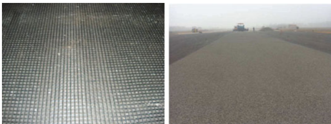
Fig. 2 Close view of glass grid and SAMI
