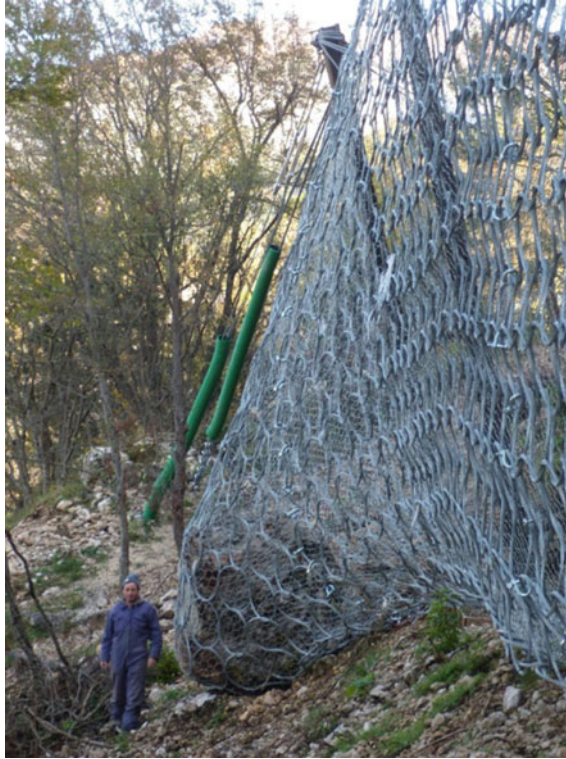
Fig. 12 The fallen block was 2.5–3.0 m 3 , and impact energy 1500 kJ, close to the Service Energy Level (SEL) of the barrier
