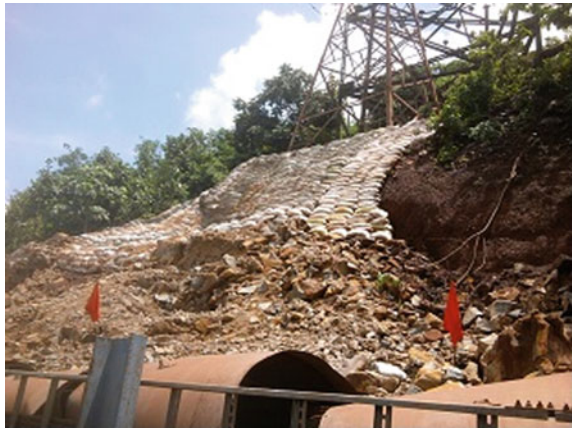
Fig. 7 Project site of 33 kV tower with damaged conveyor due to collapse of gabion and random rubble masonry wall
