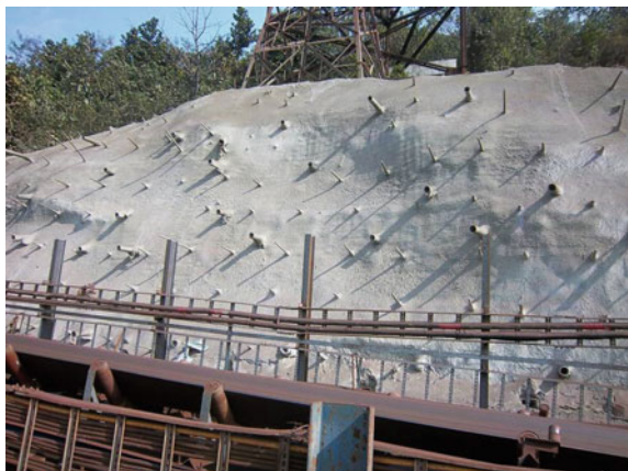
Fig. 14 Final finished slope face showing 33 kV tower at top and restored conveyor along with toe wall at bottom
