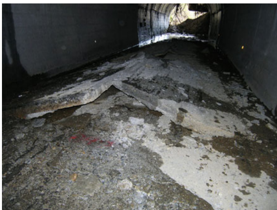
Fig. 3 Distortion of Haguro Tunnel during the earthquake
