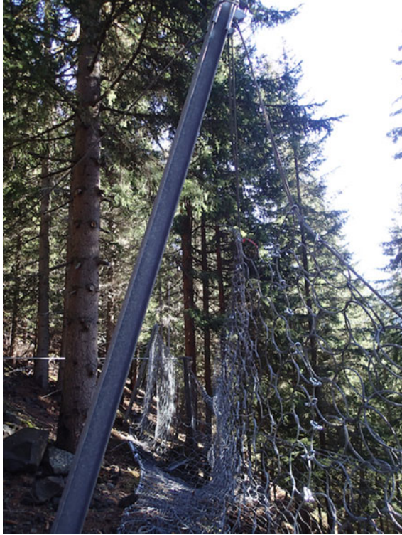
Fig. 10 The barrier was able to preserve 30–35% of residual height despite the large impact
