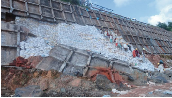
Fig. 3 Slope failure during monsoon season
