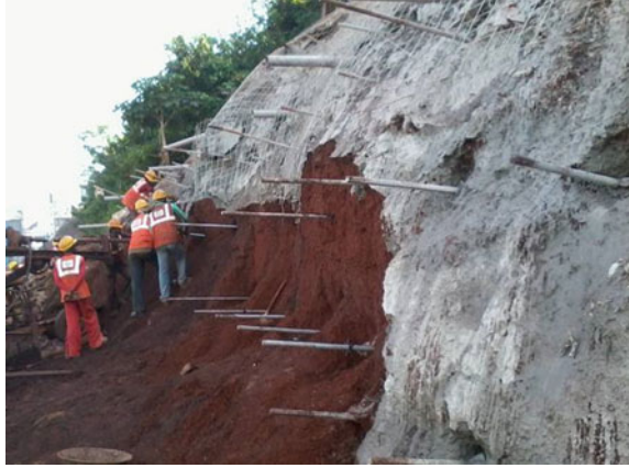
Fig. 9 Installation of grouted nails by wagon drilling machine after phase-wise debris removal from top
