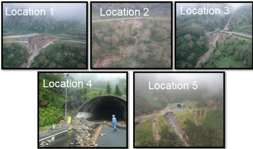
Fig. 15 Damages caused by the typhoon 10
