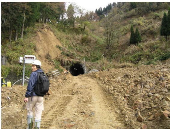
Fig. 2 Slope failure that closed the portal of Haguro Tunnel during the Chuetsu earthquake in 2004
