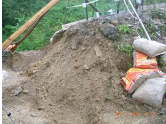
Fig. 14 Cut slope subject to artificially induced rainfall–slope failure
