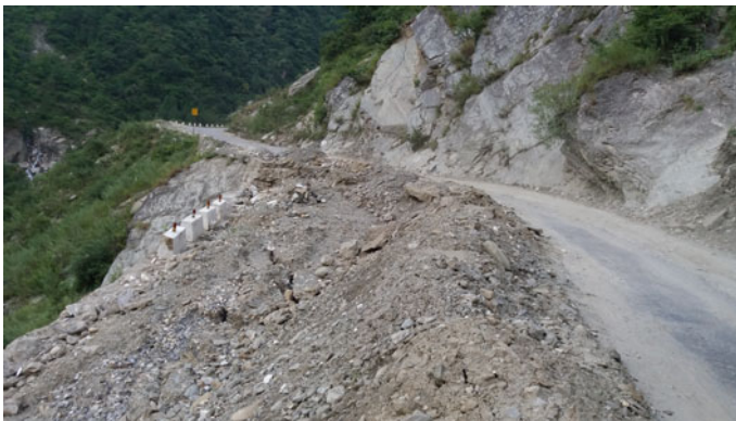
Fig. 14 Photograph showing erosion and consequent accumulated debris
