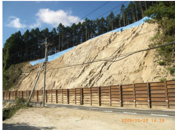
Fig. 20 Failed slope along a national highway (failure in 2009)
