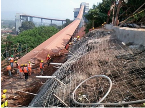
Fig. 10 Drilling and placing of perforated PVC drainage pipes and wire mesh for shotcreting layer
