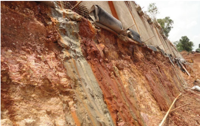
Fig. 4 Seepage water from the cut slope
