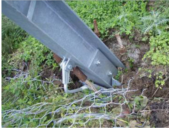
Fig. 7 Settlement of the footplates after the impact
