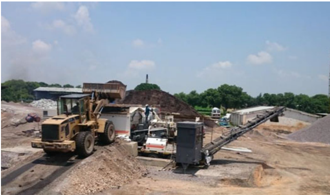
Fig. 5 A view of KMA 220 plant
