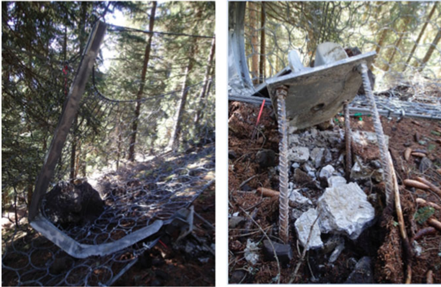
Fig. 9 Effect of the impact against the post of a 2000 kJ barrier
