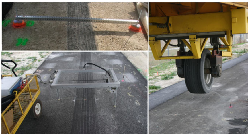
Fig. 10 ATLAS test equipment setup (right), the customized rutting measurement device for construction platforms (top left), and the laser profiler used for measuring rutting for the HMA-paved test sections (bottom left)
