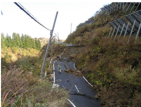
Fig. 4 Collapse of road embankment that was made of local mudstone prone to hydration and deterioration
