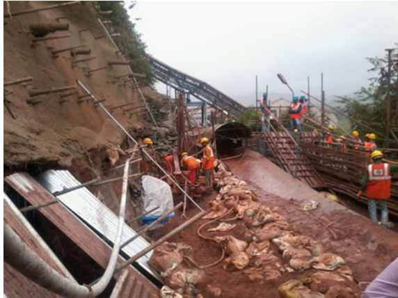
Fig. 12 Bottom debris removal and installation of vertical nails for RCC toe wall between slope toe and conveyor
