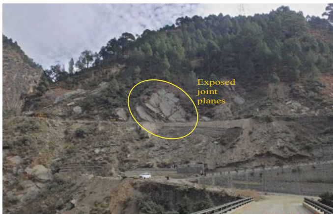
Fig. 12 Photograph showing the unfavorable dip of joints in the rock mass
