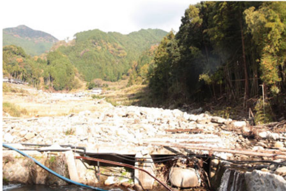
Fig. 6 Site of debris flow that affected the Chikuzen-Iwaya Railway Station of Hita-Hikosan Line
