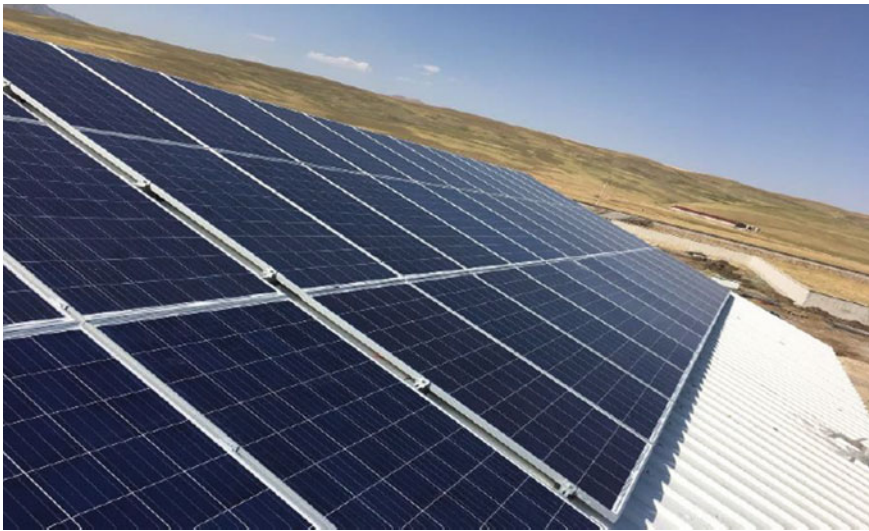
Fig. 10 Series of PV panels in a solar power plant
