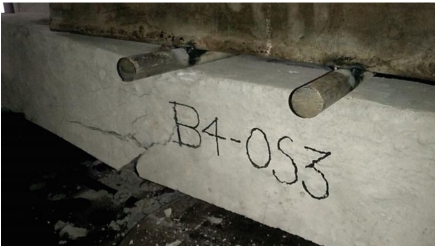
Fig. 13 Damaged beam 4 (OS 3) with visible cracks
