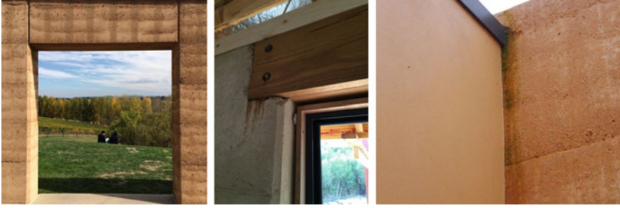
Fig. 8.11 Examples of stains on wall caused by bad execution and/or design ( Photo Rodrigo Rocha 2015 )
