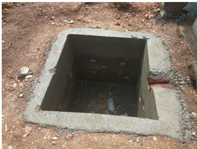
Fig. 7.5 FEC sanitary soak pit in Kudapura village, Challakere, Karnataka state, India
