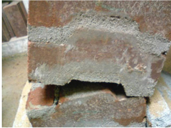
Fig. 14.7 Failure in block
