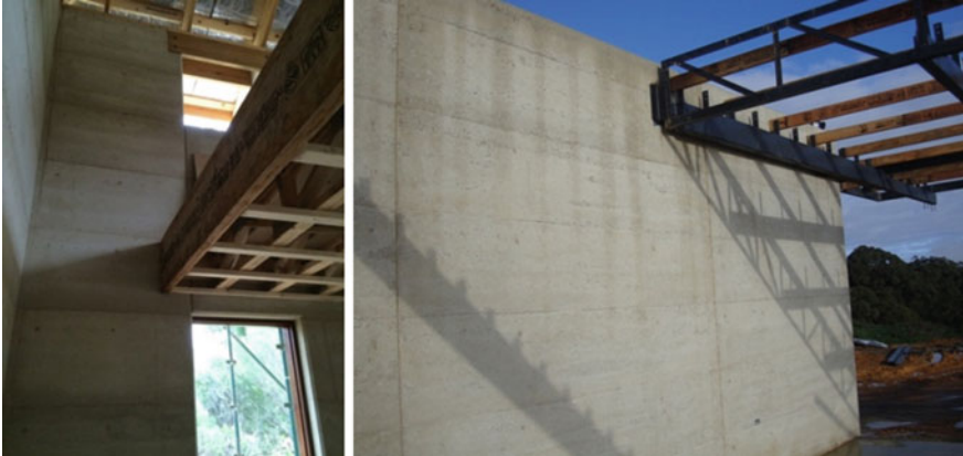
Fig. 8.7 Example of connections to timber floor and steel roof beams (Photos Oliver Petrovic 2014)
