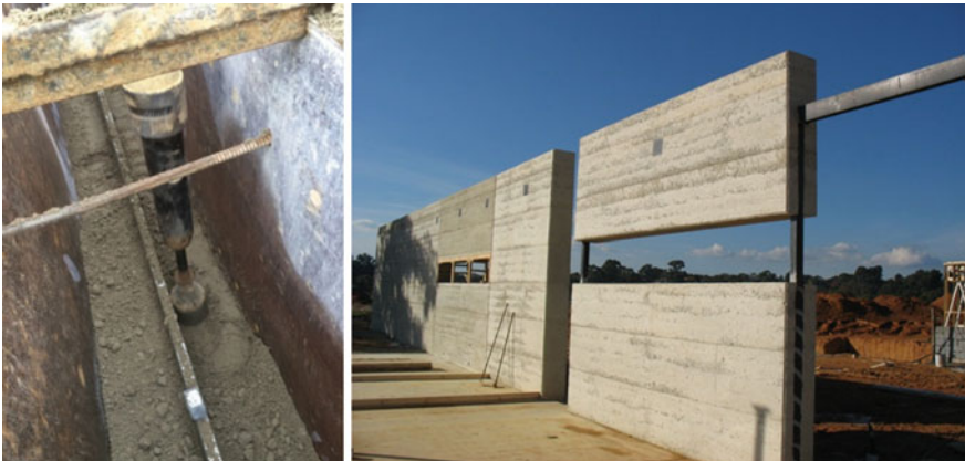
Fig. 8.8 SRE building process over T-shaped steel beam and built-in steel column (Photos Rodrigo Rocha and Oliver Petrovic 2014)
