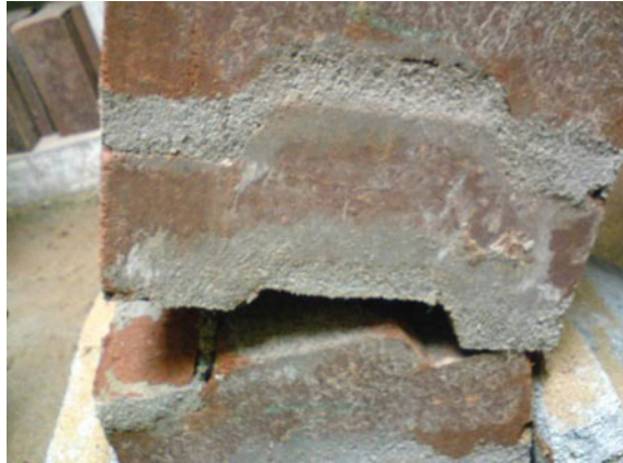
Fig. 14.7 Failure in block
