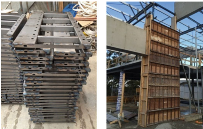
Fig. 8.2 Manufacturing of the steel framework and its use in the construction process ( Photos Rodrigo Rocha 2015)
