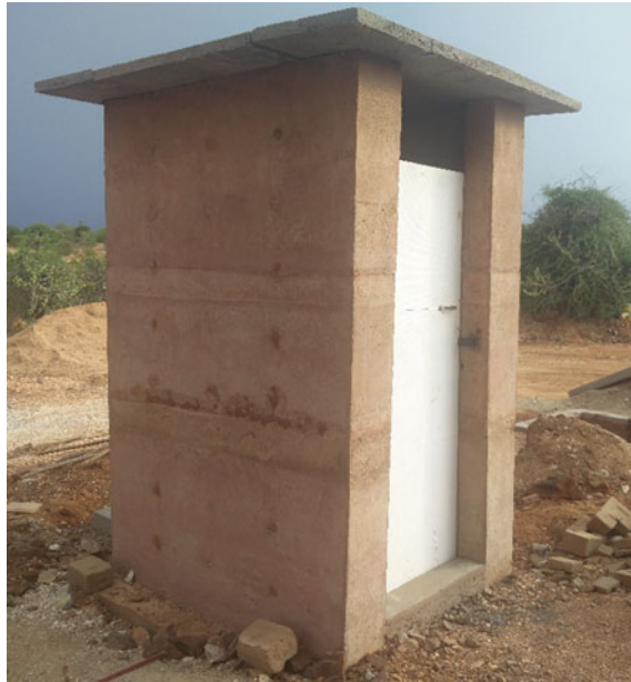
Fig. 7.4 FEC sanitary unit in IISc Campus, Challakere, Karnataka state, India
