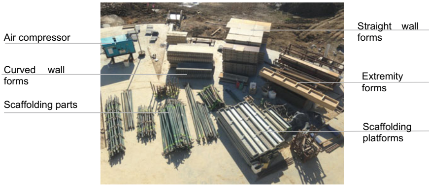
Fig. 8.1 Equipment used in the building process of the stabilized rammed earth ( Photo Oliver Petrovic 2014)
