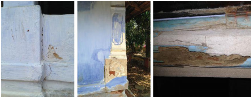
Fig. 37.8 Plaster cracks, plaster detachment, improper treatment (cement plugging) of termite infested wood (L-R)
