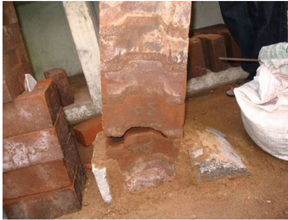
Fig. 14.6 Failure at bond–mortar interface
