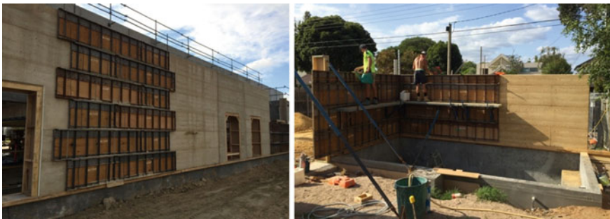
Fig. 8.10 Examples of use of formwork and aluminium platforms resting on cantilevered brackets in the SRE walls building process (Photo Rodrigo Rocha 2015)
