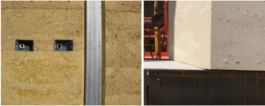
Fig. 8.6 Detail of built-in electrical installation, example of built-in steel column and contrast with corten steel ( Photo Rodrigo Rocha 2015 )
