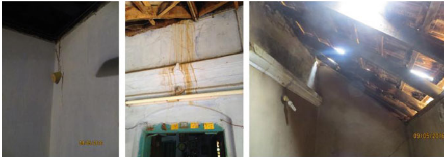
Fig. 37.7 Termite attack on walls, damages in roof that causes issues in the wall structures (L-R)
