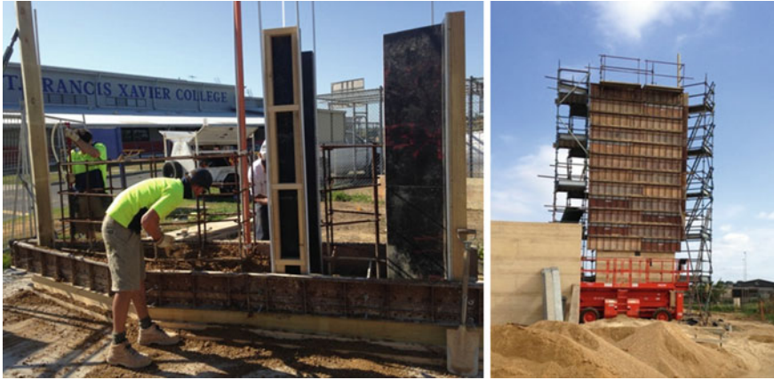
Fig. 8.3 Example of the building process of a 12-m-tall reinforced SRE tower ( Photos Oliver Petrovic 2014)
