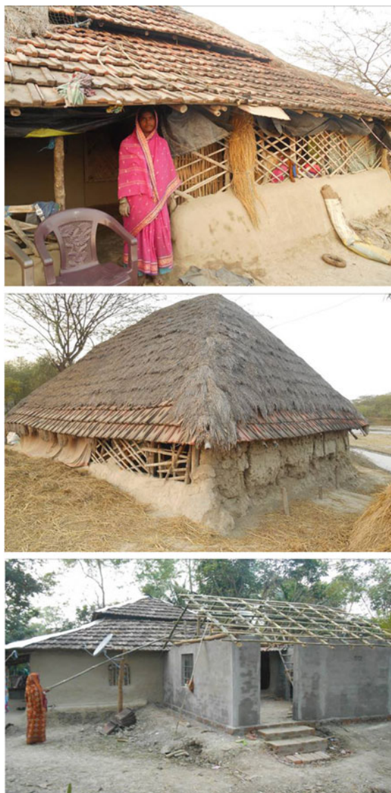
Fig. 13.8 Houses of beneficiaries in the Sundarbans [bottom picture–house of Chandi Das name changed]
