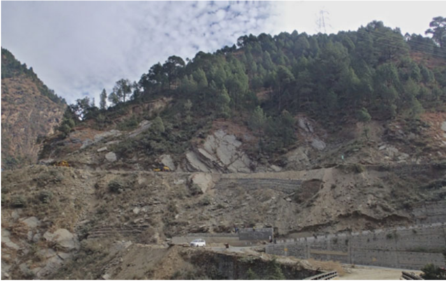
Fig. 19.1 Landslide zone at Birahi
