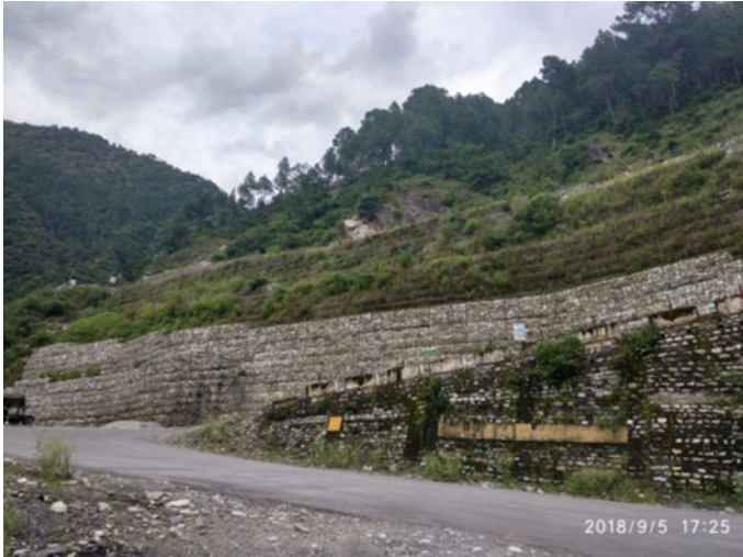
Fig. 19.16 Current status of retention system at Birahi
