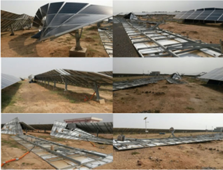
Fig. 21.1 Photos indicating the extent of damage witnessed due to heavy wind
