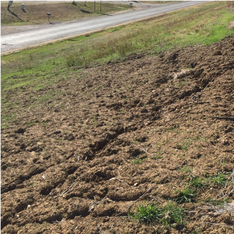
Fig. 2.2 Typical desiccation cracks observed in slopes consisting of expansive soils in the Dallas-Fort worth region
