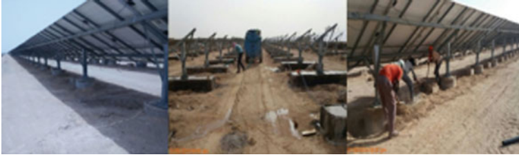
Fig. 21.2 Photos indicating the repair, rectification, and maintenance of foundation and module mounting structure
