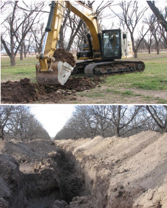
Fig. 9.10 Excavation to modify soil profile. (Photo source: Texas A&M AgriLife Research Center at El Paso)
