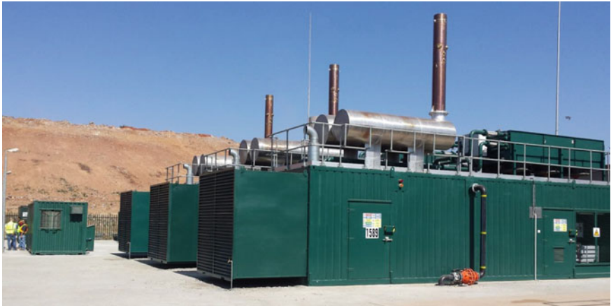
Fig. 7.17 Landfill gas to power facility in Johannesburg (Infrastructure News 2016)
