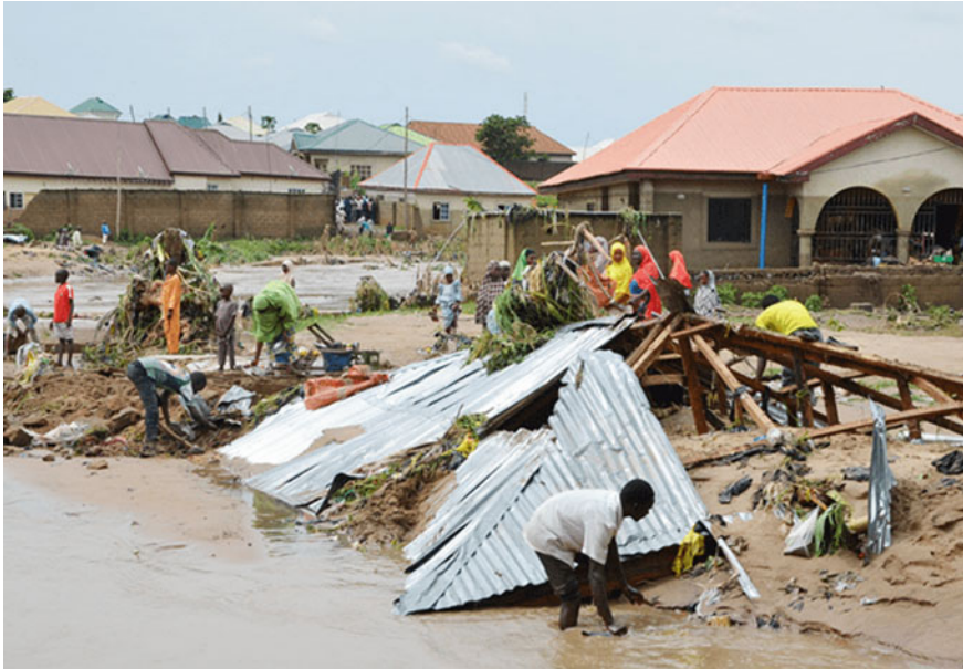
Plate 10.1 Windstorms removing roof-top of a house. Source https://www.google.com.ng/search?biw=1366&bih=659&tbn=isch&sa=1&q=flood+in+Lagos&oq=flood+in+Lagos&gs_l=psyab.3..012j0i24k1l2.80339.83338.0.83789.11.10.0.0.0.0.741.1870.2-1j0j2j0j1.4.0.....0...1.1.64.psy-ab..7.4.1867...0i67k1.mI9mqLrQOxw
