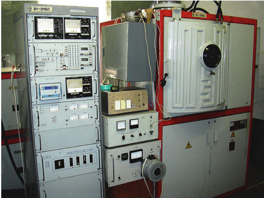
Fig. 2 Upgraded installation of microarc vacuum ion plasma coating VU-2MBS-m
