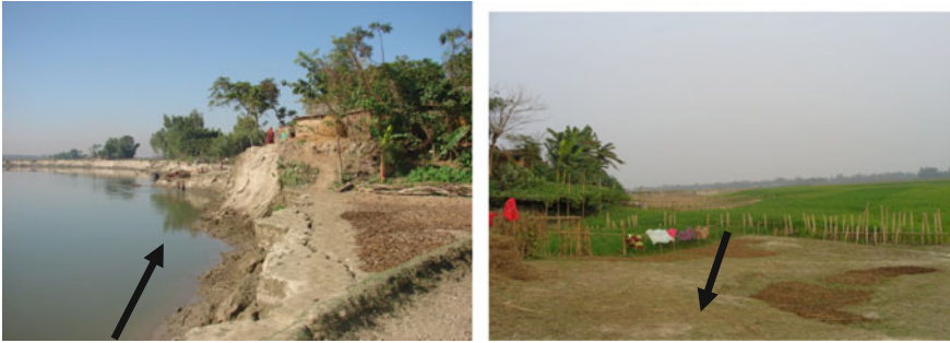
Fig. 11 River before the construction of bamboo bandalls in the left and that of after the flood in the right of the photographs
