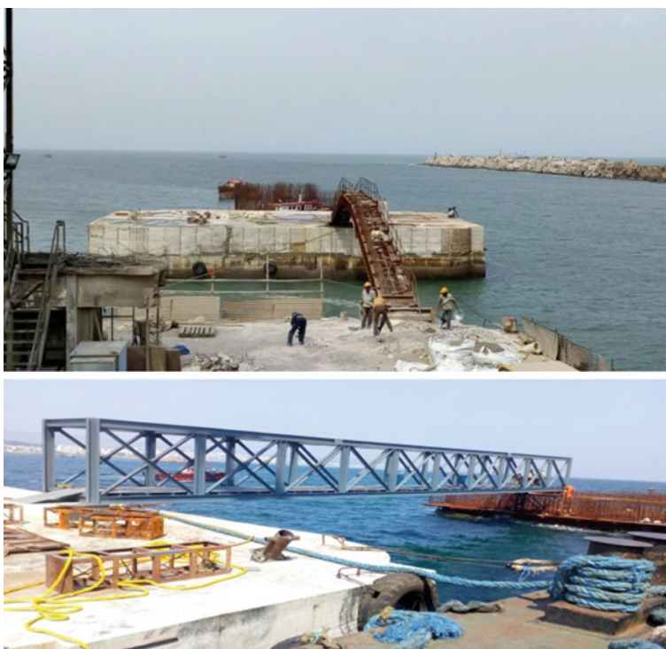
Fig. 11 View after completion of deck slab (top) walkway between berthing and mooring dolphin (bottom)
