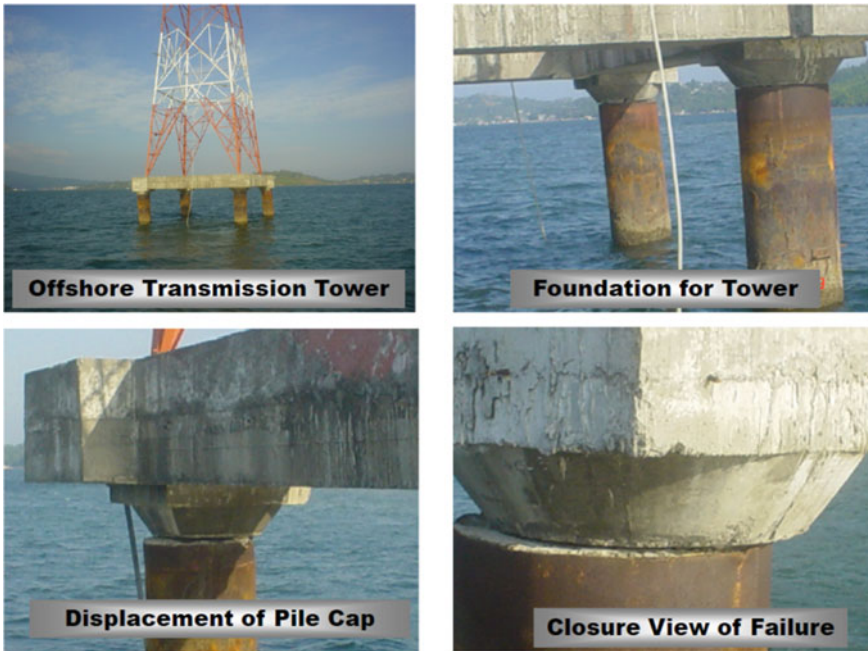
Fig. 9 Displacement of pile cap in offshore transmission tower
