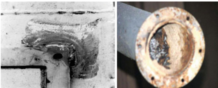
Fig. 1 Burning at the welded joint and dust explosion in pipe [7]
