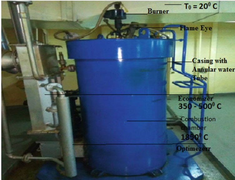
Fig. 1 Rx4 Auxiliary boiler
