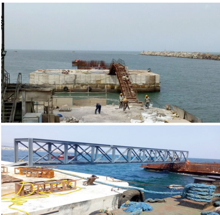
Fig. 11 View after completion of deck slab (top) walkway between berthing and mooring dolphin (bottom)
