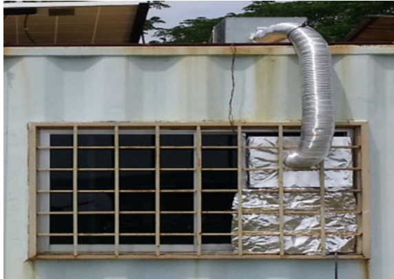
Fig. 10 Experimental setup for solar-powered ventilation
