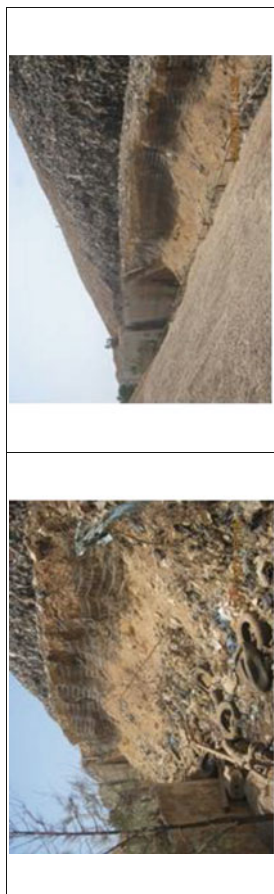
Fig. 3 Current situation of the collapse of the peripheral wall
