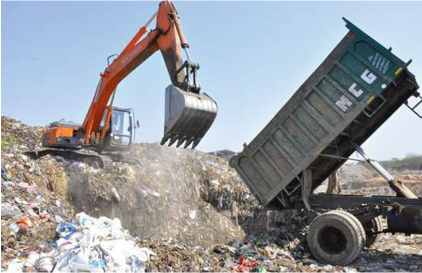
Photo 8 Fresh waste unloaded and moved back to form windrows above the unloading spot
