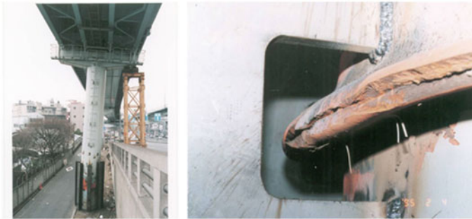
Fig. 1.3 Ductile fracture of a circular hollow section pier after elephant's foot buckling in the 1995 Kobe earthquake (Gao et al. 1998a, b)
