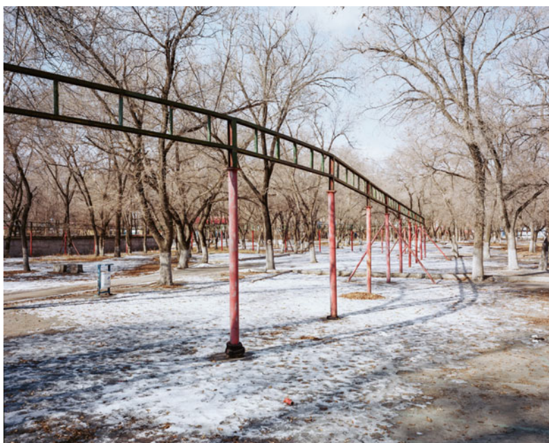
Fig. 11.4 A rusted roller coaster rail stands abandoned in Hong'an Park
