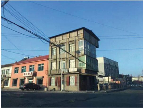
Fig. 13.13 The typical worn-out space in the town: damaged roads, defects of curbs, lack of rubbish bins, wooden packages, and temporary windows
