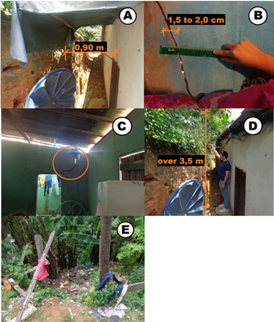
Fig. 3. Conditions of the houses in very high risk: (A) Distance of the house from the slope on the crest; (B) and (C) Cracks found in both houses; (D) House with more than 3.50 m built below the crest of the slope; (E) Dumping waste on the face of the slope.
