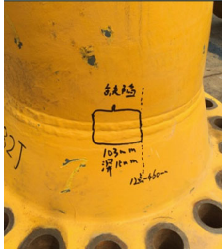
Fig. 3. The defect found by phased array detection
