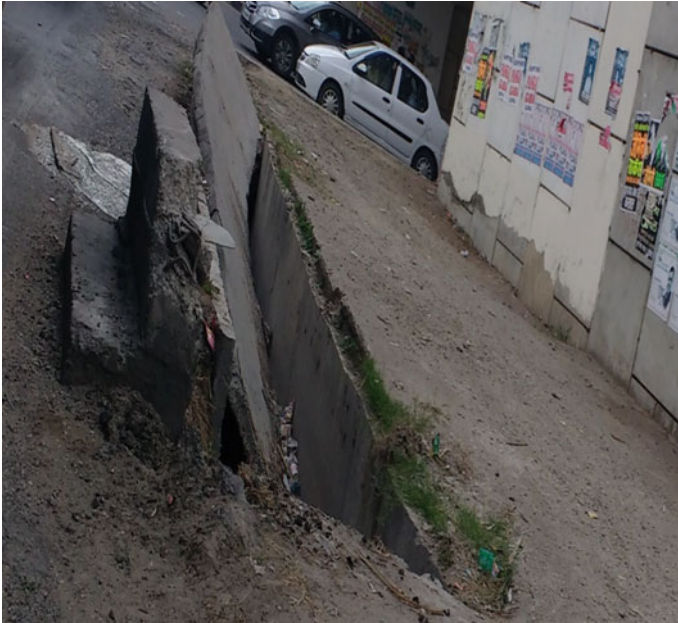
Fig. 2 Covering slab lying in the drain
