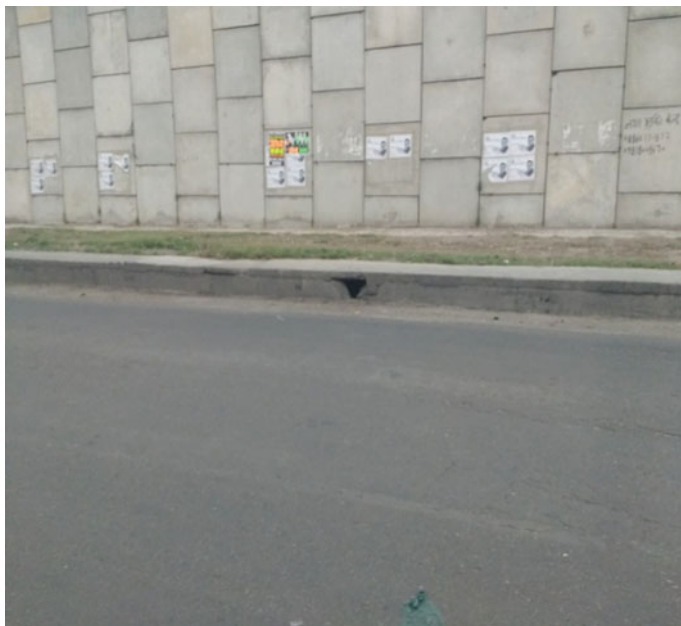
Fig. 4 Improper entry point of drains
