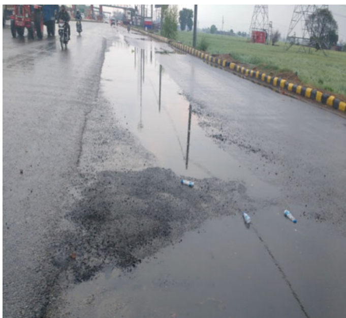
Fig. 5 Adverse slope resulting into stagnation of water on the road
